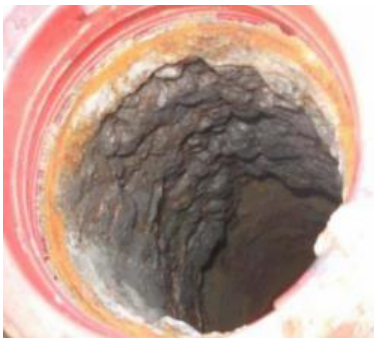
Fig 1. Scale deposited in downhole tubular (Tao Chen et al. 2017)
